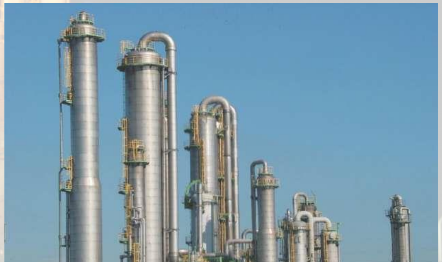
Distillation units to separate phenol and propanone
